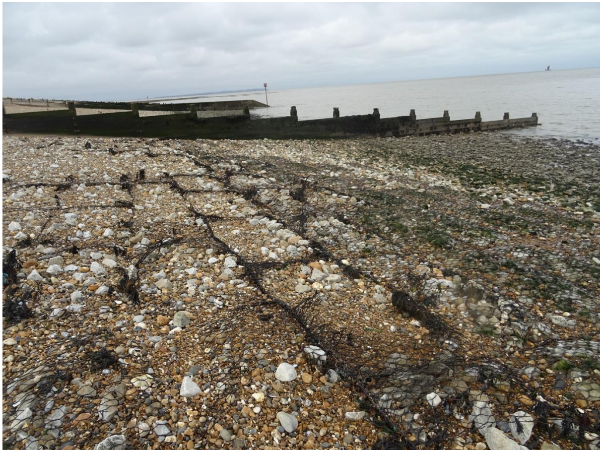
FIGURE 8-7 WIRE MATTRESS EXPOSURE AT EASTERN END OF SWALECLIFFE (2016)
