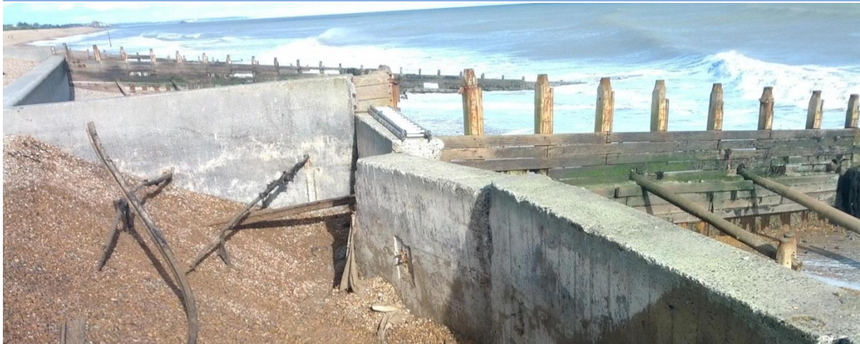
FIGURE 6-2-16 DILAPIDATED GROYNES LOW BEACH AND SEA WALL FAILURE AT KINGSDOWN (2013)
