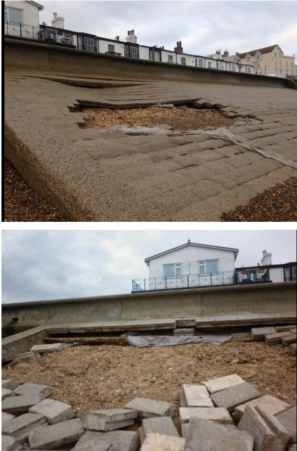
FIGURE 8-9 SEA WALL FAILURE IN HERNE BAY SECTION H AFTER ONE TIDE 9 (LEFT) AND AFTER TWO TIDES (RIGHT)
