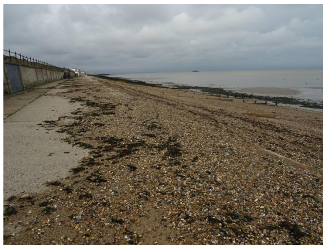
FIGURE 6-2-13 EVIDENCE OF OVERTOPPING ON TO THE PROMENADE (HERNE BAY, 2016)
