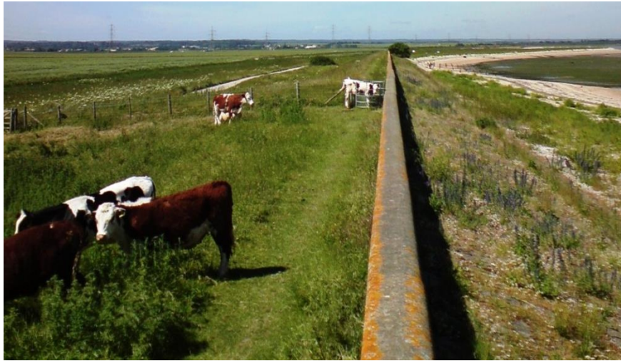
FIGURE 1-9 VEGETATED BLOCK WORK APRON AND WAVE RETURN PROFILE WALL ON CLAY BUND, BACKED BY GRAVENEY GRAZING MARSH (2008).
