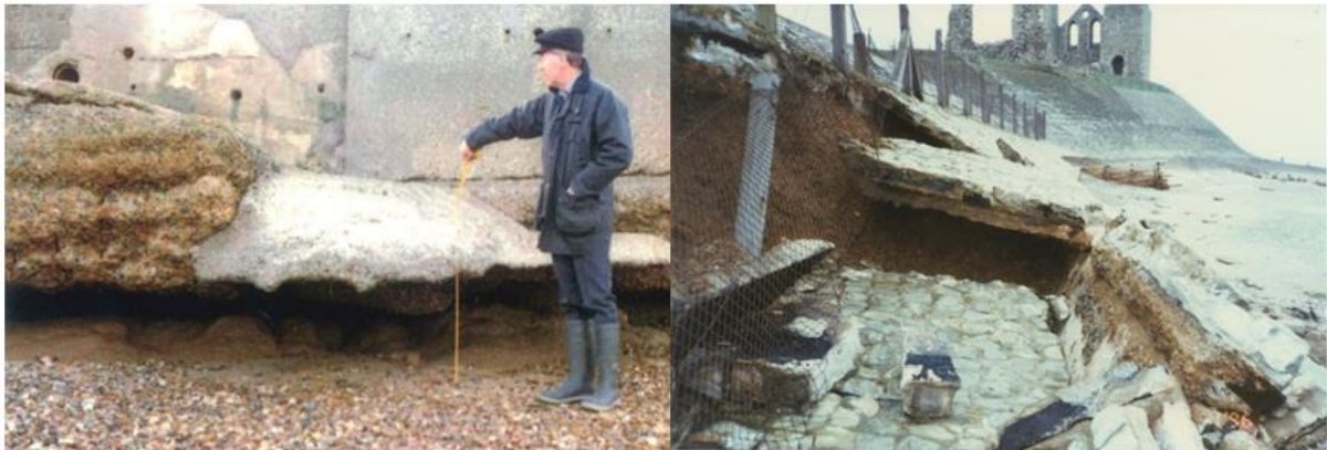
FIGURE 6-2-17 EXAMPLES OF UNDERMINING AT TANKERTON (LEFT) AND RECVLVER (RIGHT) (BOTH PHOTOS 1999)
