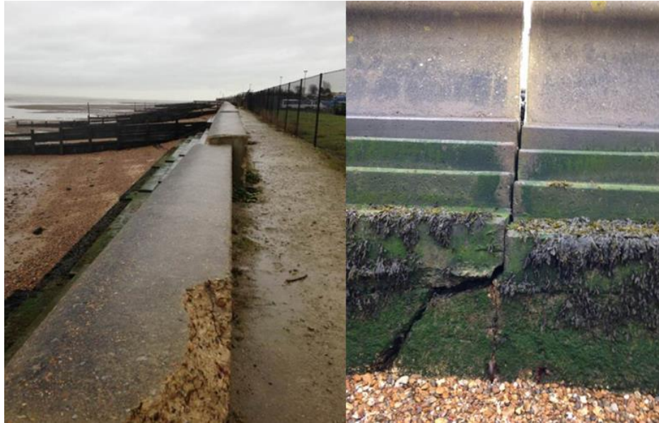
FIGURE 6-2-18 FAILURE OF A SEA WALL AT ALL HALLOWS DUE TO SLIDING/TOPPLING OF DEFENCE SECTIONS (2015)
